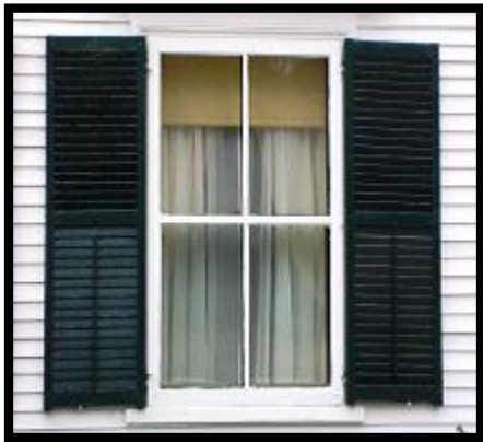
A well-proportioned 2/2 storm window installed over a 2/2 double-hung sash window.
