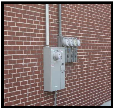
Example of appropriate placement of electrical meters on a secondary elevation
