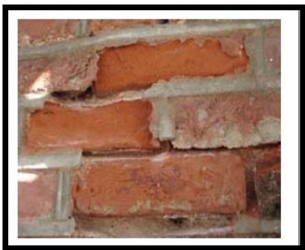
This building has been damaged by the application of Portland cement in mortar joints, which trapped moisture in the bricks and caused the face to deteriorate and pop out. The Portland cement was a harder material than the brick. Always uses mortar that is softer than the historic bricks.
